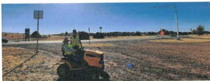
Joe Fairchild and Fay Hume looking over a job well done on east median.
